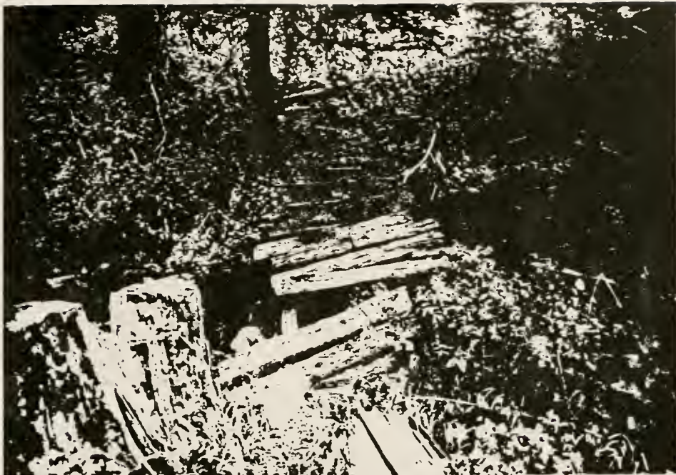
Figure 267. Stuart-Schultz Cabin 24PA410), west view below cabin showing foot bridge across Pine Creek that leads to Diversion Dam (Structure #164).
